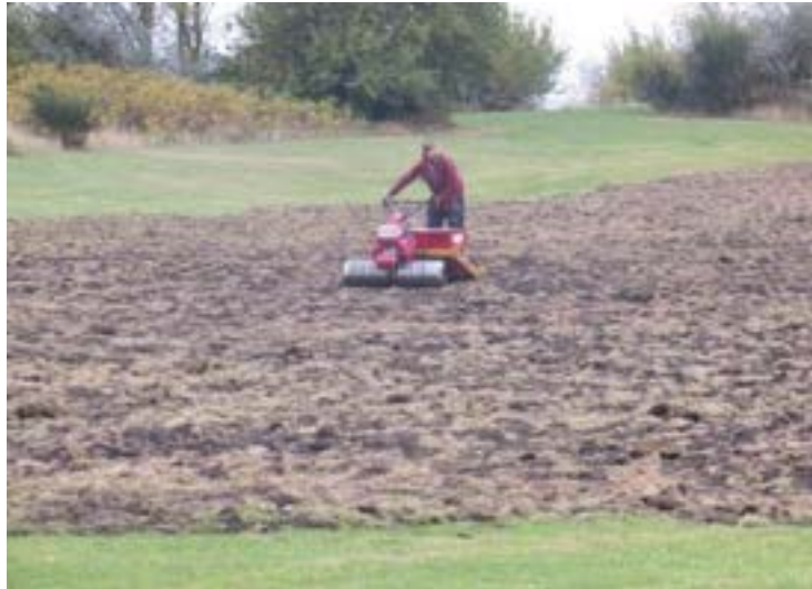
Figure 3. A roller used by contractors to help break up the soil after a power harrow had been used.
